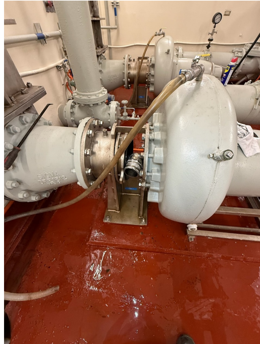
Male cam lock found in pump station
